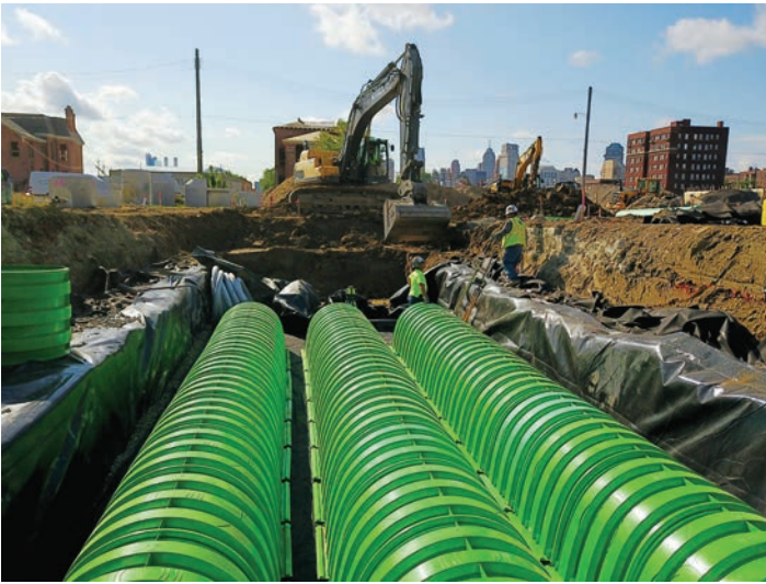
A liner was necessary to prevent infiltration of contaminants from the surrounding soil.
