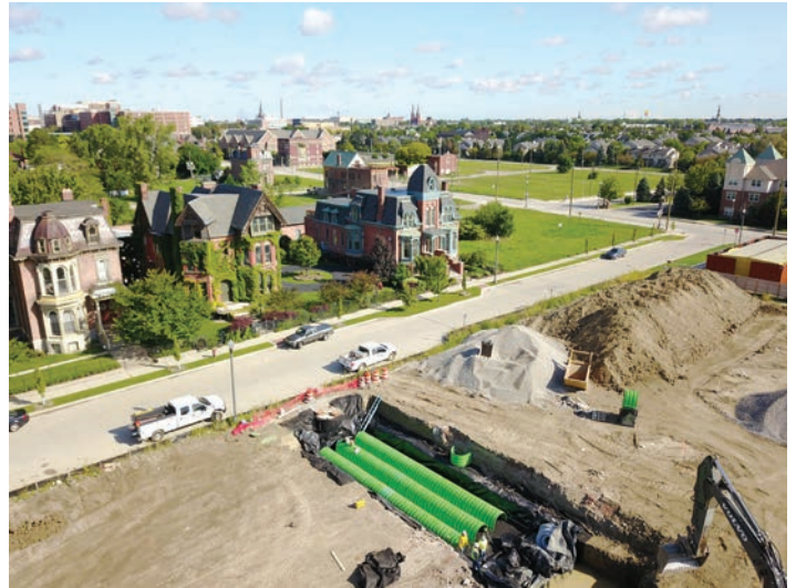
20 individual Triton systems were implemented to facilitate the limited space.
