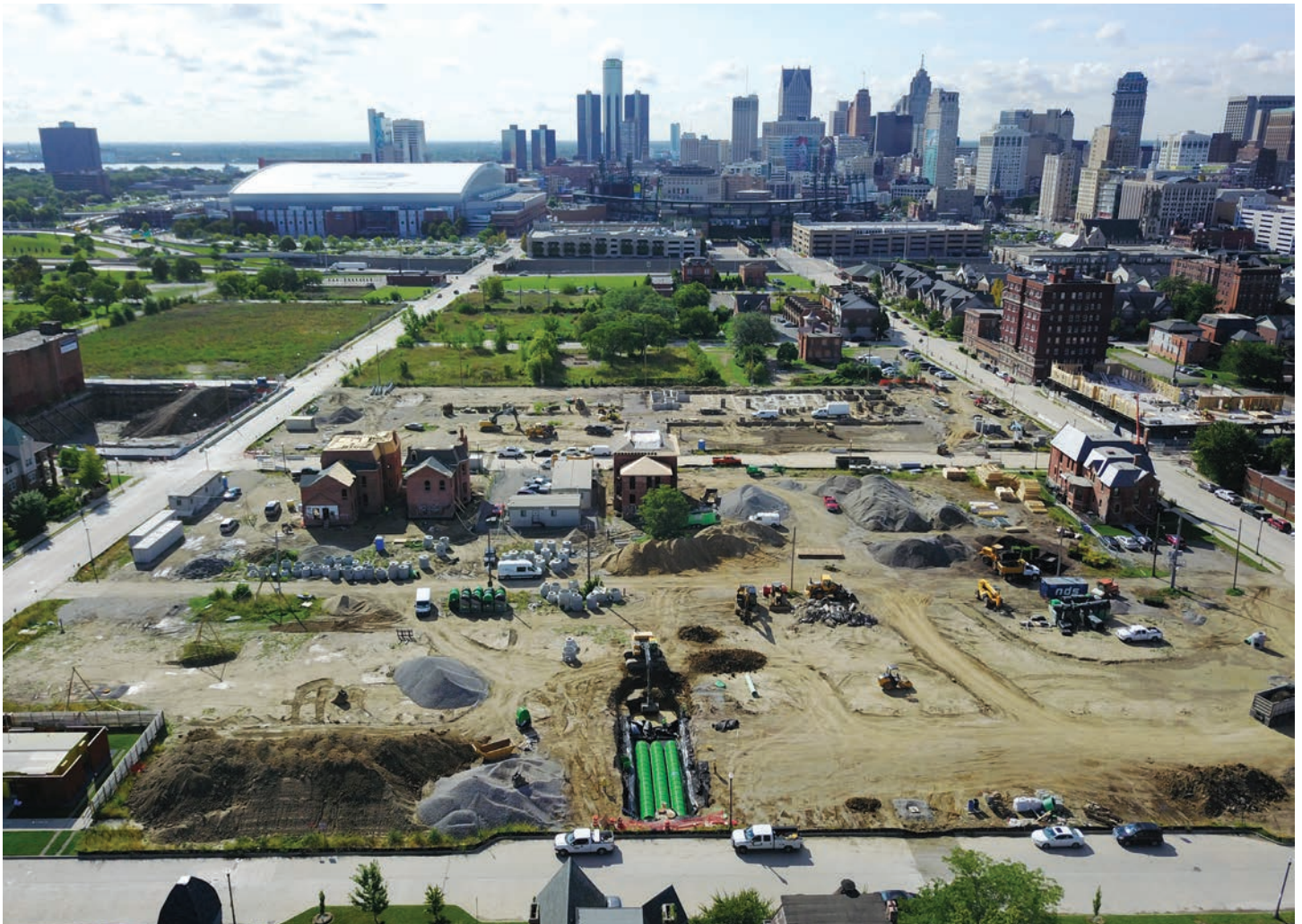
Triton systems will efficiently manage stormwater in Brush Park, an up-and-coming neighborhood
